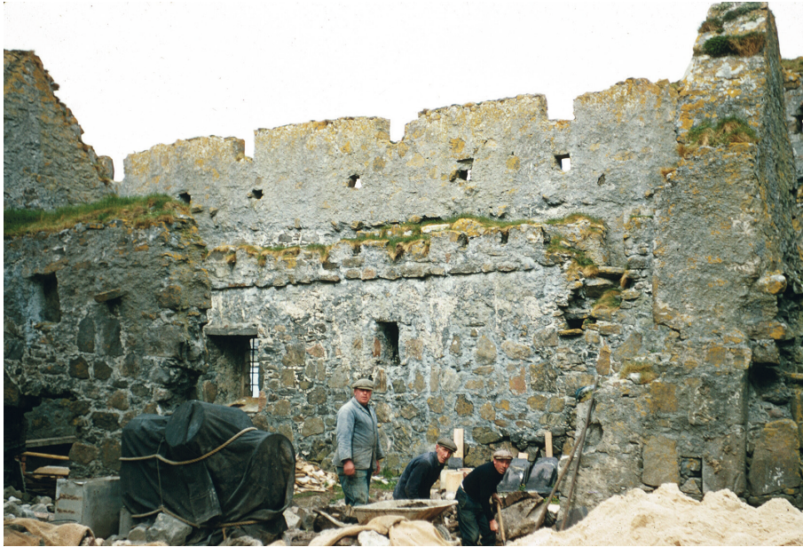
ILLUS 9 Areas of the west wall exposed during the reconstruction of the hall (Macneil Collection 1960s, S434, © Crown Copyright: HES)
